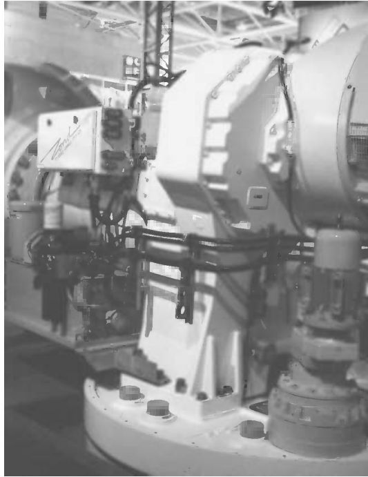
Figure 6.28 Integrated gearbox on Zond Z-750 turbine. (The gearbox is mounted on a circular nacelle bedplate, with the hub to the left and generator at the rear. An electrically driven yaw drive can be seen beneath the generator)
