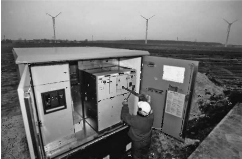
Figure 10.4 Transformer and switchgear of 1.5 MW wind turbine, MV switchgear is on the right LV switchgear on the left. Reproduced by permission of NEG MICON
