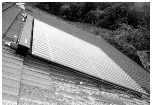
The solar hot water tubes installed on the roof provide an ample supply for much of the year.
