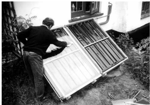
Paul and Judith Otto's entirely home-made solar water heating system cost them just under £800 for materials at 1994 prices. Self-installing a factory made system can save around half the cost of one which is professionally installed.
