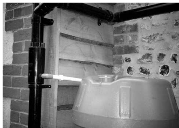
The rainwater collection system at Tim and Maddy Harland's house. When the tank is full rainwater is automatically diverted to the downpipe by the filter device.
