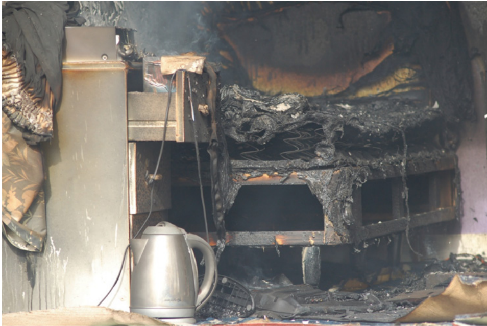
Figure 5.2 The aftermath of a fire.
