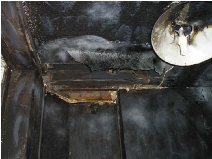
Figure 5.11 Fire scene reconstruction – ceiling.
