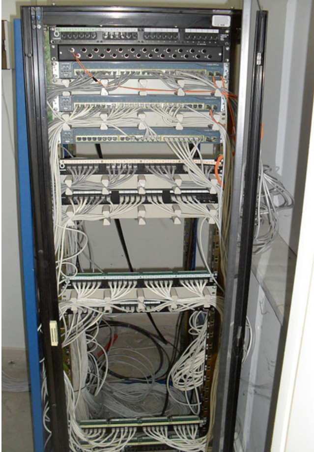
Fig. 3.7 Rack with patch panels
