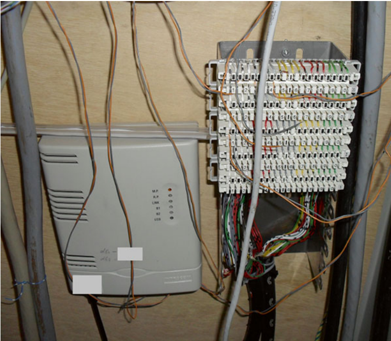
Fig. 3.4 Small office main distribution frame and CPE
