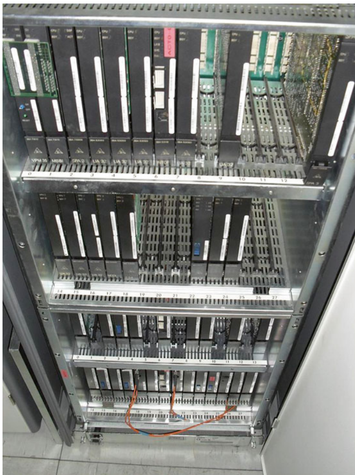
Fig. 1.2 The front side of the PBX
